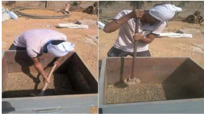
Fig 4. Preparation of bottom most layer filling and compacting subgrade and granular subbase
