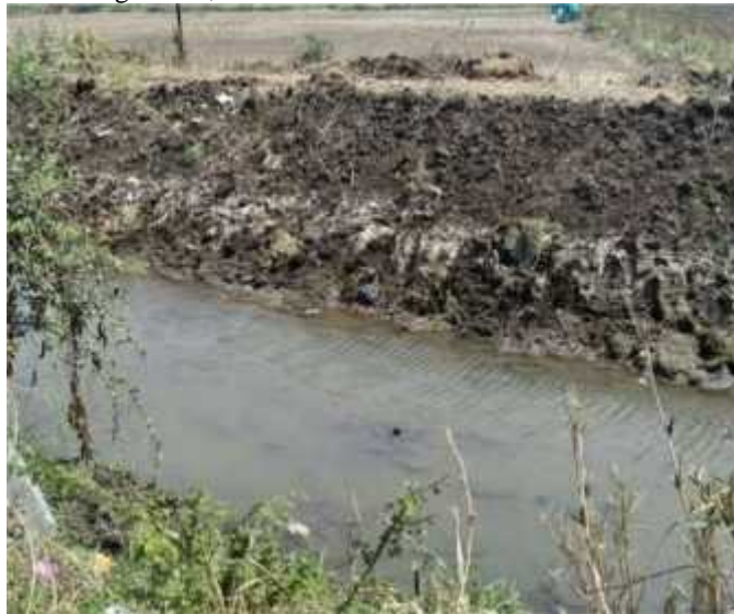
Fig. 1. Canal Slope Failure
