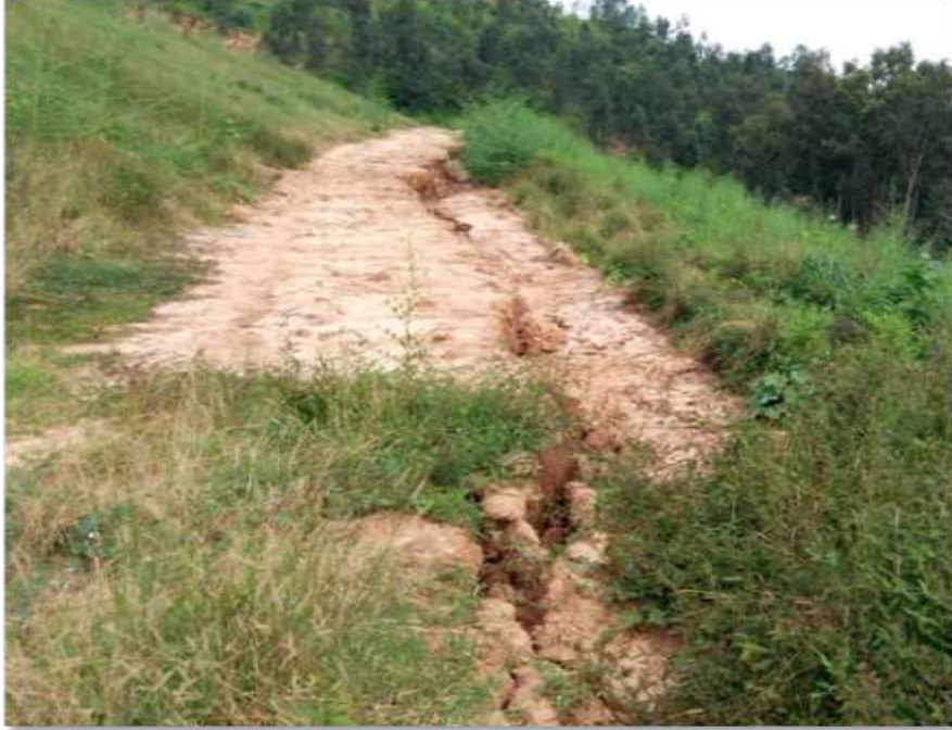
Fig.4. Subsidence Stretch at Upper Bench above Starter Dam
