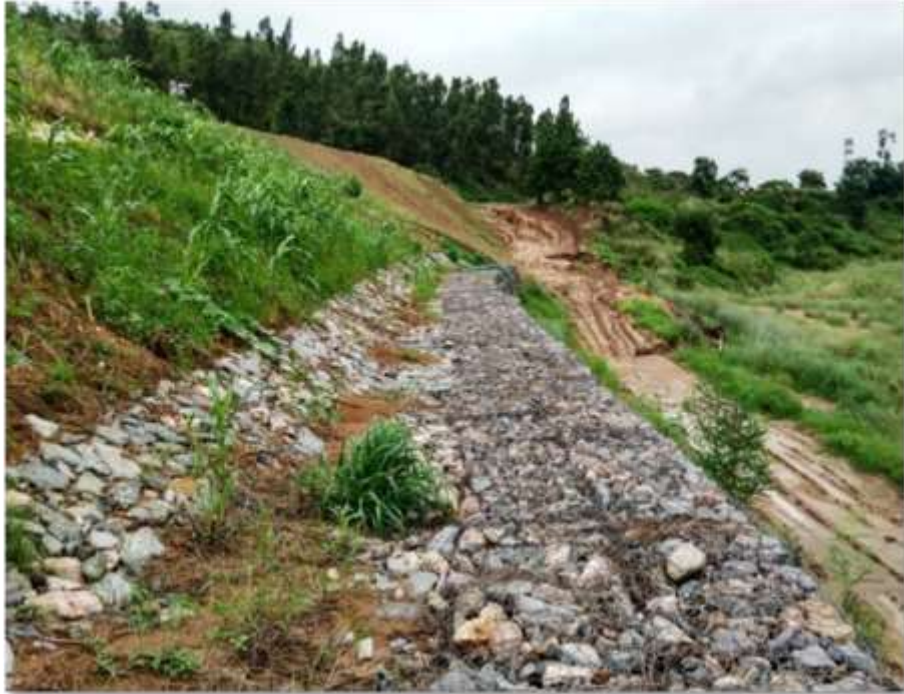
Fig. 12. Gabion Wall at Toe of Starter Dam and Grown Vegetation on Slope
