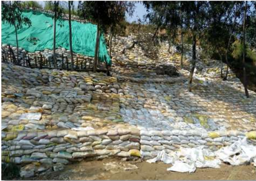
Fig.5. Seepage Zone of Starter Dam Toe & Downstream Slope with Sand Bags
