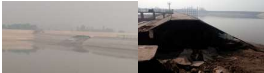
Fig. 1. Some photos of breached portion of embankment
