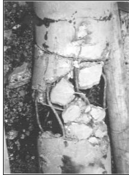
Fig.3. Failure of pile with 2m lateral ground displacement during the 1964 Niigata earthquake
