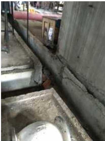
Fig.1. Cracks in the seal oil foundation
