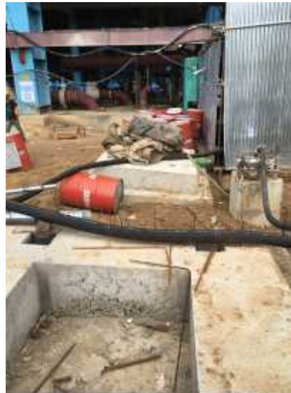
Fig.2. Tilted foundation due to settlement
