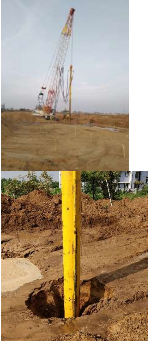
Fig. 7. Depth vibrator in action & Subsidence in the form of conical crater due to compaction
