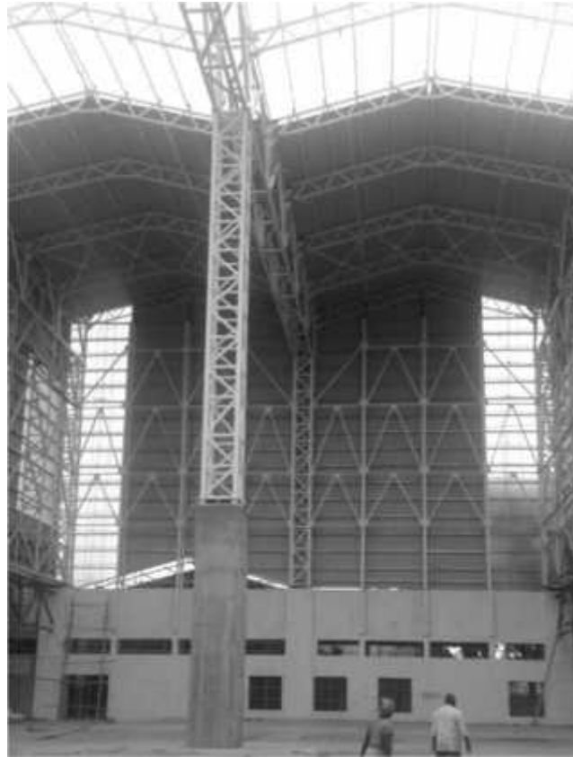
Fig. 7. Site photos showing the erected steel structure on renovated RC column over the Underpinned foundation
