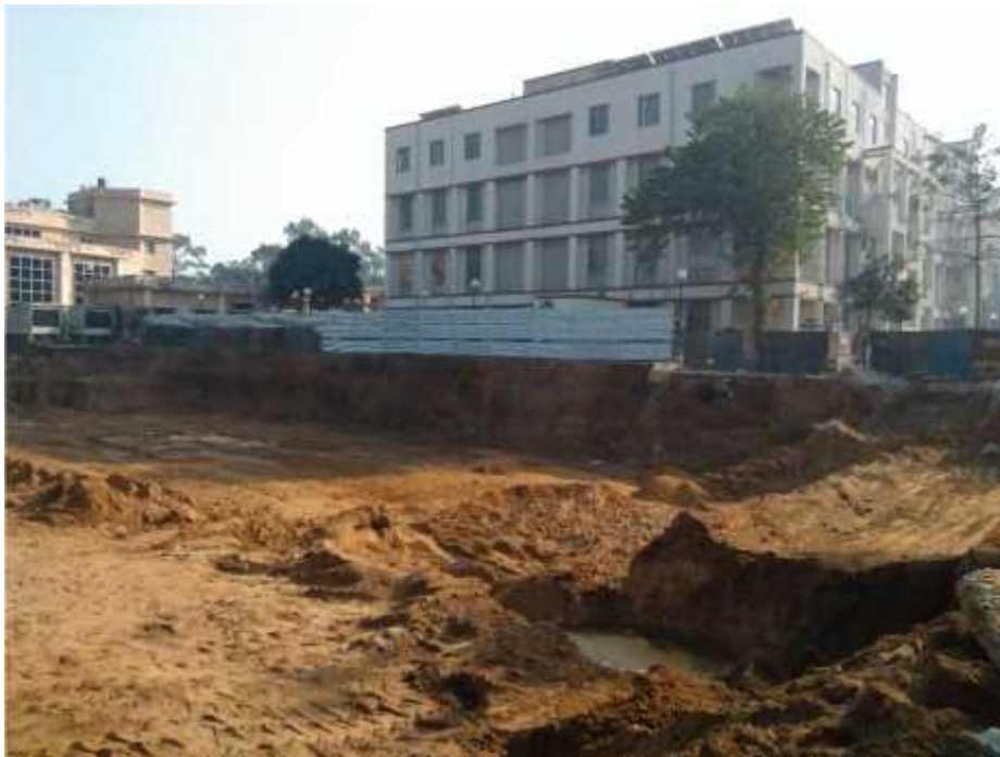
Fig. 1. Unsupported excavation adjacent to an existing building.
