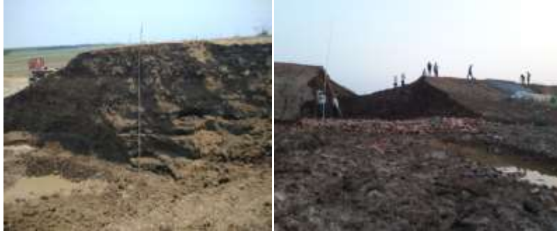
Fig.2. Photos showing breached sections of summer storage (SS) tank
