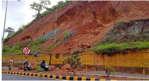
Fig.1. Landslide on national highway connecting IDC Verna to Loutolim,Goa.
