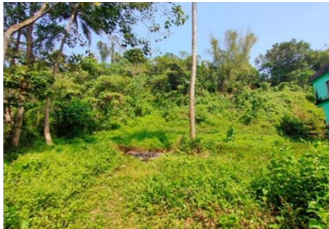
Fig.3. Present condition of Kormala slope
