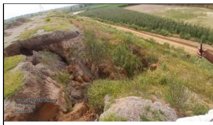
(c) Insufficient growth of vegetation
