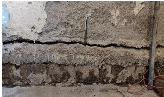
Fig .1. Settlement of Wall in the Courtyard of Building
