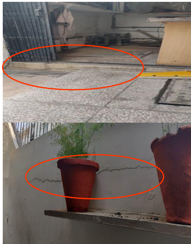
Fig.2. Photographs of cracks in the building
