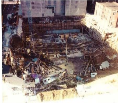
Fig.1. Collapsed site (sighted from west)
