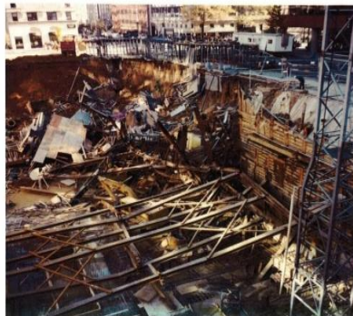
Fig.2. Collapsed site (sighted from east)
