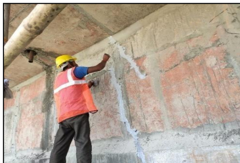
Fig.14. Cracks sealed with putty
