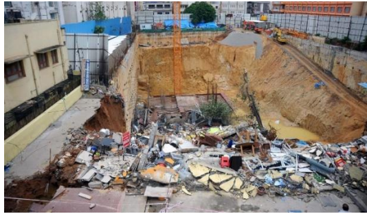
Fig.8. construction error at site.
