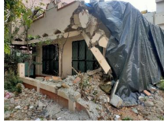
Fig.4. Damages caused to adjacent building.
