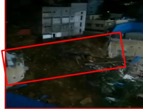
Fig.7. Reason for soil displacement
