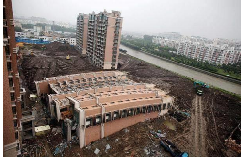
Fig.11. Failed structure at Shanghai
