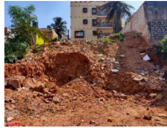
Fig.4. Soil movement from beneath the foundation
