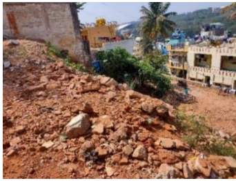
Fig.3. Elevation of collapsed building site
