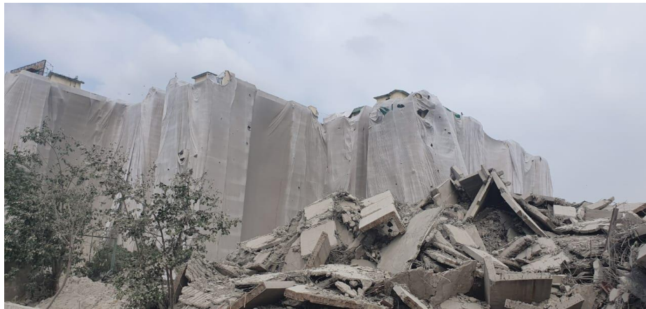
Fig.14. The photograph of Aster-2 after the demolition of the Supertech Twin tower
