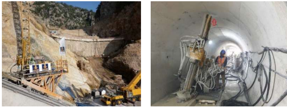
Fig. 14. Mobile platforms for drilling and grouting works on slopes with the exposed bulkhead behind (left) and working in gallery (right)
