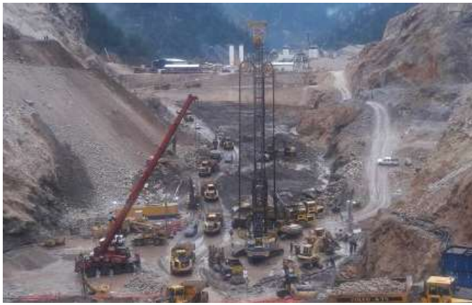
Fig. 13. Imposed congested working zone with dumpers, access road to reservoir, stockpile area through the bulkhead working area
