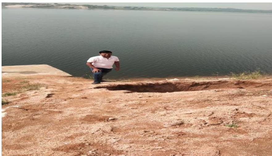
Fig 1(b). Cavity on the upstream face of the reservoir.
