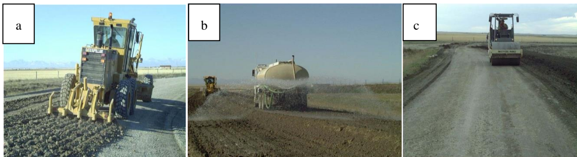
Fig. 6. a) Scarifying of road surface, b) Application of Terrazyme, c) Rolling and compaction
