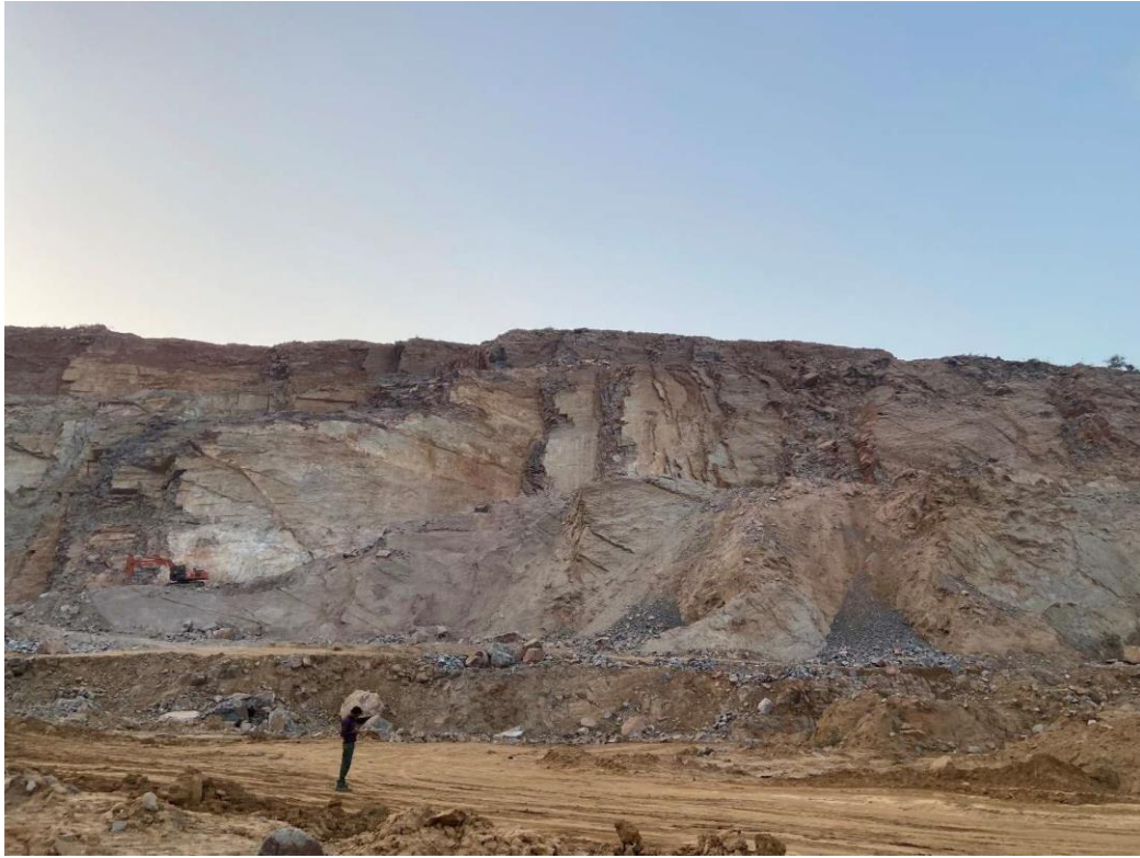
Fig. 4. Photograph of a stretch at the project site showing exposed rock cut face.
