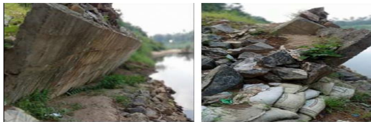
Fig. 4. Laterally displaced retaining wall
