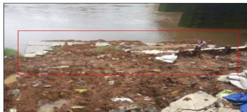
Fig. 2. Collapsed retaining wall
