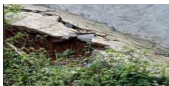
Fig. 5. Cracks due to vertical settlement
