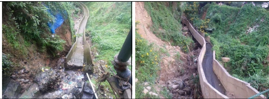
Fig. 5. Condition (eroded and broken) of side drains adjacent to affected slide
