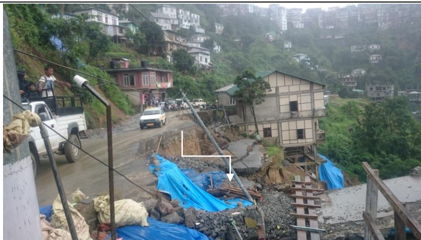
Fig. 4. Sinking / sliding of National Highway
