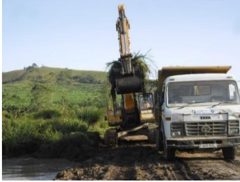
Fig. 2. Removal of vegetation, muck and unsuitable soil from the bed of Swamp
