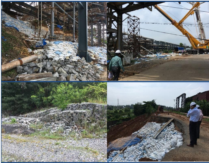
Fig. 1. Photographs showing the pattern of ground destabilization at site.
