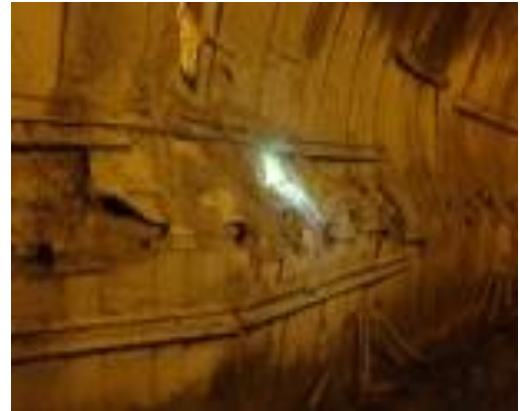
Fig.10. Bending of ribs due to squeezing in HRT Face-2
