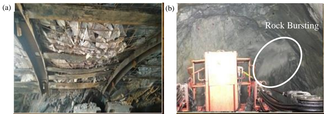
Fig. 1. Rock bursting observed from (a) crown of HRT Face-4 and (b) right wall of HRT Face-3
