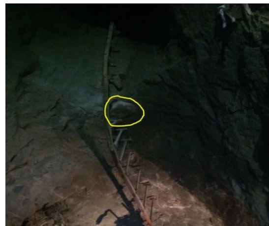
Fig.8. Hanging rock chunk at the crown portion in delivery main-2.
