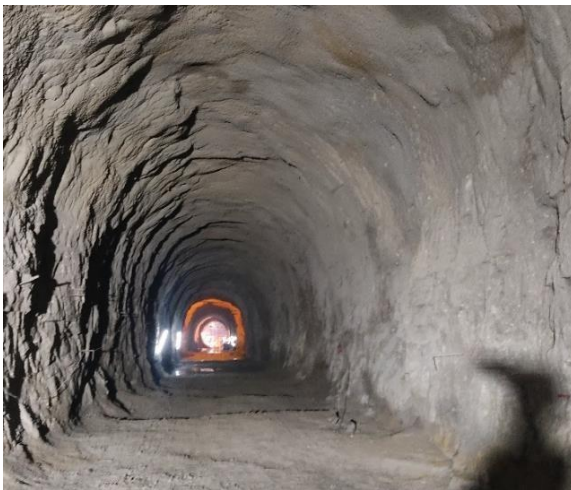
Fig. 3. View of full excavated delivery main tunnel-4, junction point of horizontal and vertical portion is also shown
