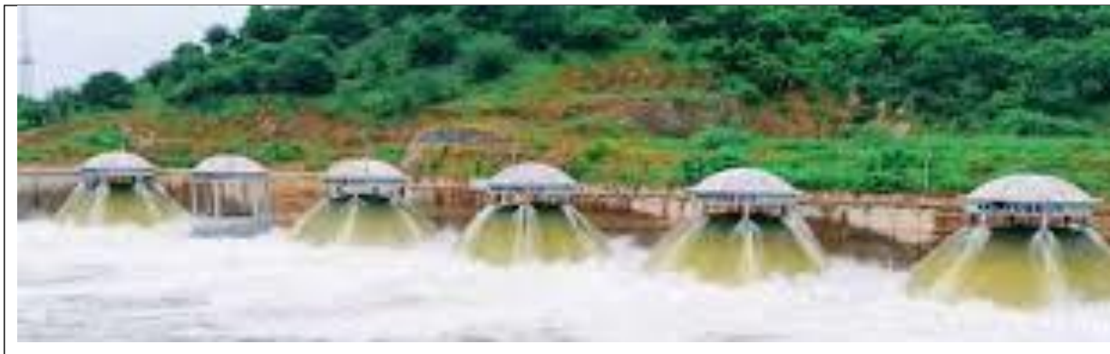
Fig. 10. Panoramic view of delivery mains in the operational stage (lifting of water)
