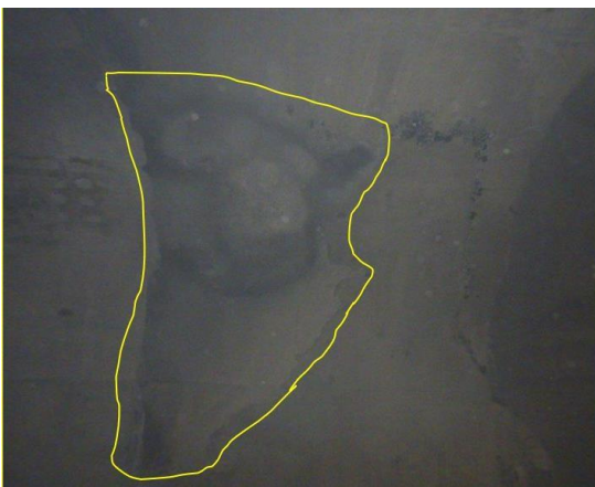
Fig. 7. Rock damage portion on the right crown of delivery main-1 and treated with shotcrete.
