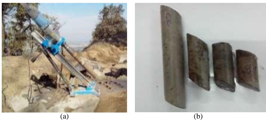
Fig. 2. In situ coring of the specimen (a) portable coring equipment and (b) preserved samples
