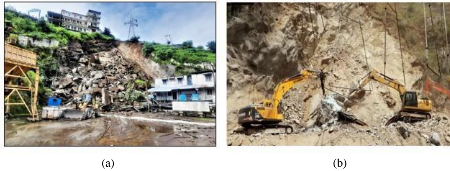
Fig. 1. (a) Collapsed tunnel portal at Tapovan Vishnugad hydroelectric plant, Uttarakhand, India (2021); (b) Under-construction tunnel collapse on the Jammu-Srinagar National Highway near Khooni Nallah, in Ramban, India (2022)
