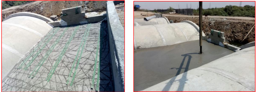
Figure 9 Installation of arch and filling of CLSM, along with laying of soil reinforcement (EcoStrap™)
