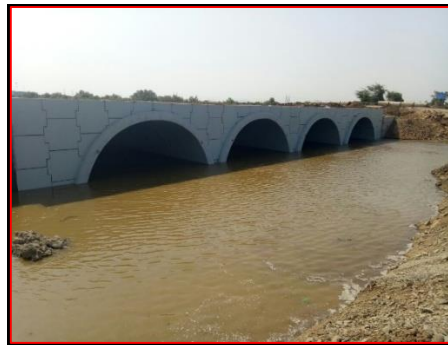
Figure 10 Completed Arch bridge structure with TechSpan and head wall with Reinforced Earth wall
