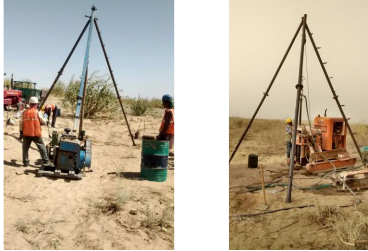
Fig. 2. Boreholes in progress. Photo on left illustrates soil boring in progress using mechanized shell and auger. Photo on right illustrates rock coring being done using hydraulic rotary rig
