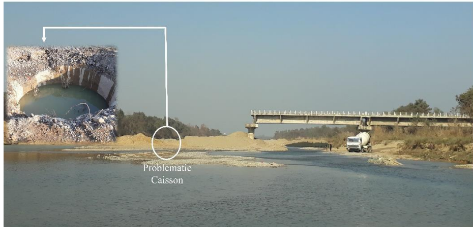
Fig.1. Problematic bridge construction due to caisson sinking issues in Tinau River, Nepal
