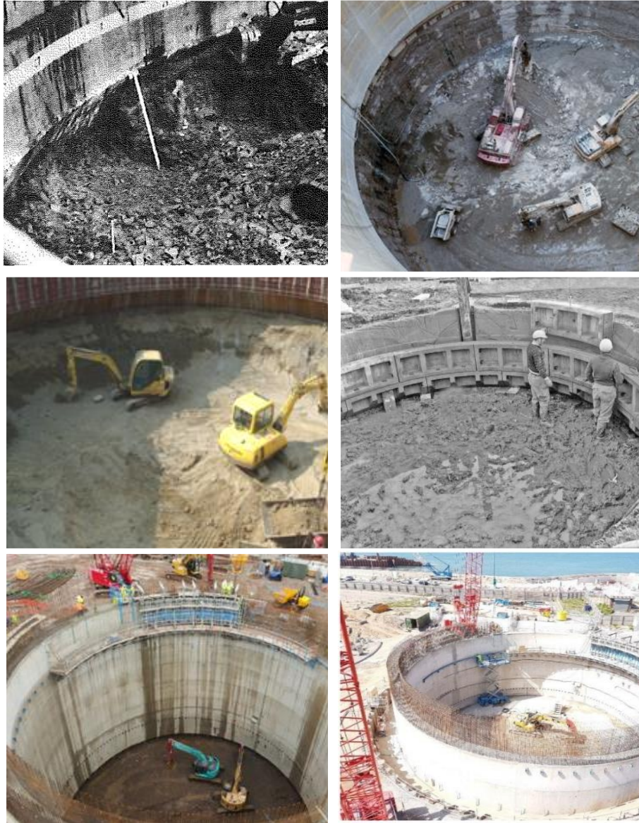
Fig. 1 Large diameter caisson for launch and reception pits for tunnel boring machines and underground units like pumping stations, storm water tanks, storage and attenuation tanks (Nonveiller, 1987; Allenby et al., 2009; Yao et al., 2014; Royston et al., 2016; Sheil et al., 2018)
