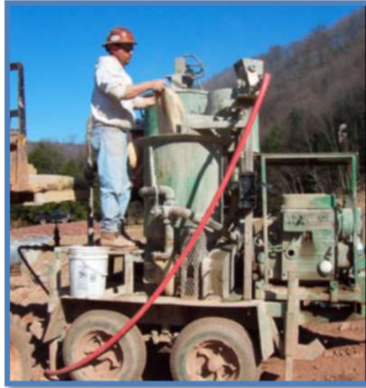
Figure 7.10. Mobile grout plant capable of being moved around a site near the injection point.
