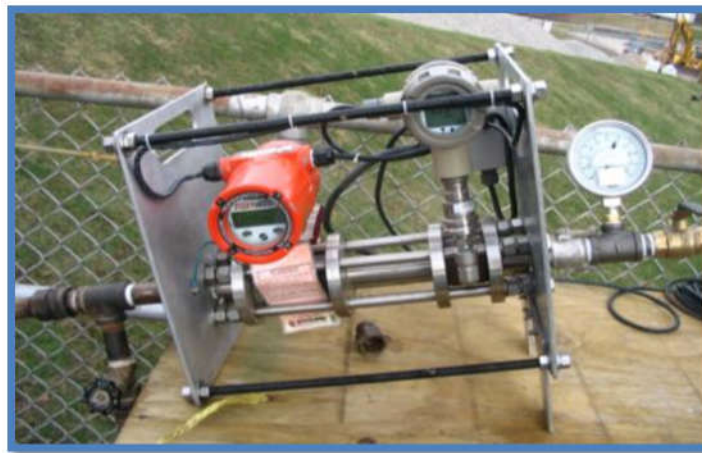
Figure 7.9. Electronic system for flow and pressure readings used in pressure testing.
