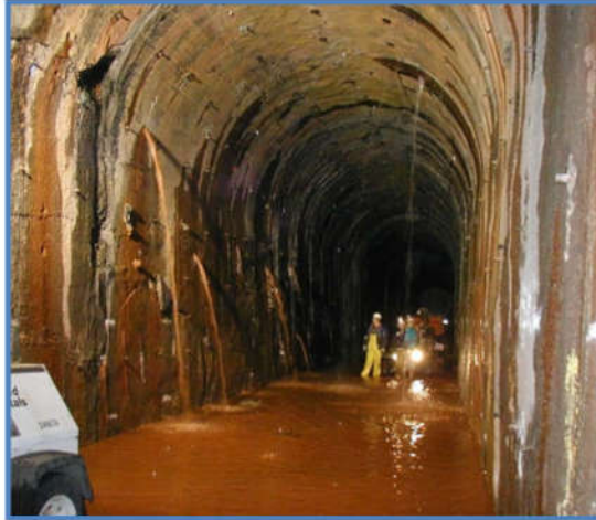
Figure 2-2. Seepage in Tunnel
