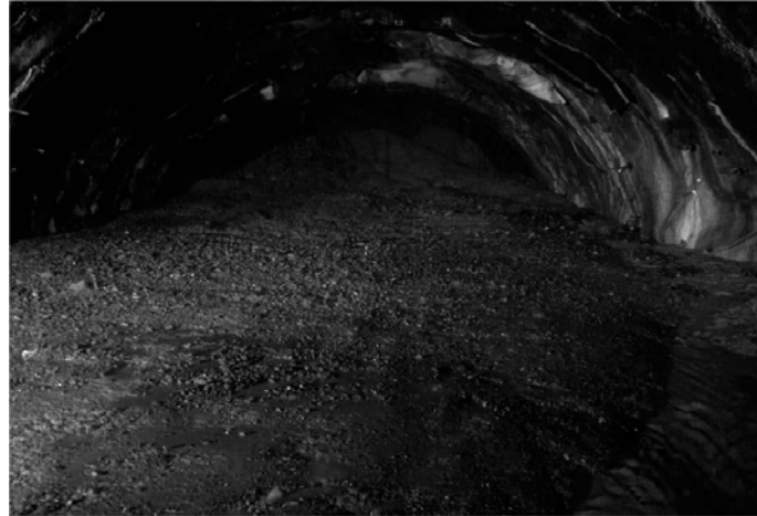
Figure 3 Flow of clay matrix along with highly disintegrated and weathered rock mass from tunnel face at Ch. 2077m (Rao & Sharma, 2014).
