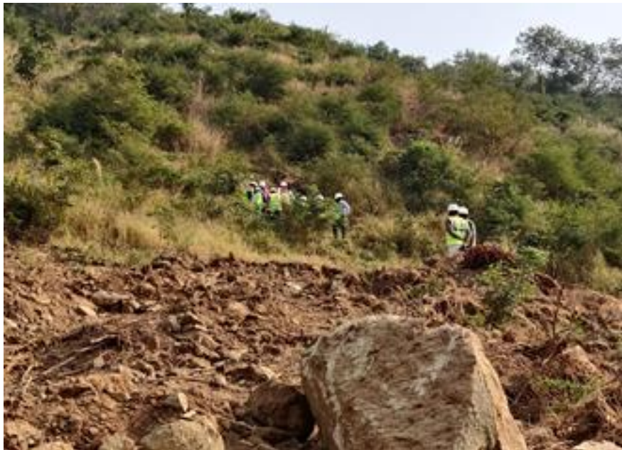
Fig.21 - Slope cutting preparation to start construction of T1 tunnel of BBB railway project
