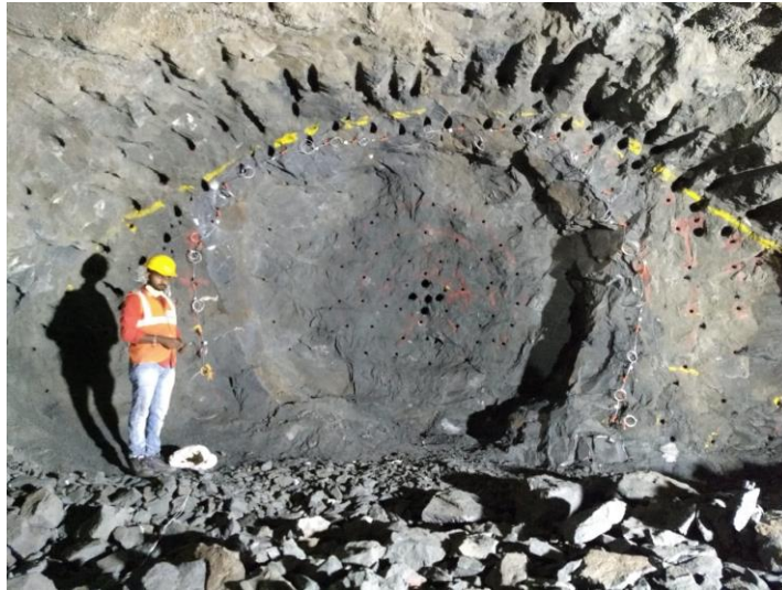
Fig.25 - View of excavated inner blast rings during controlled blasting in Adit-1 of Mumbai metro
