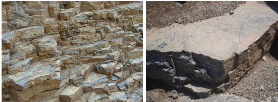
Fig. 112. Close up view of the 3 sets of joints (J1, J2, J3) in Dolomitic rock on left abutment
