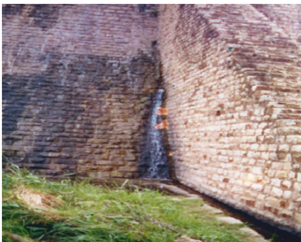
Fig. 43 Seepage through masonry dam
