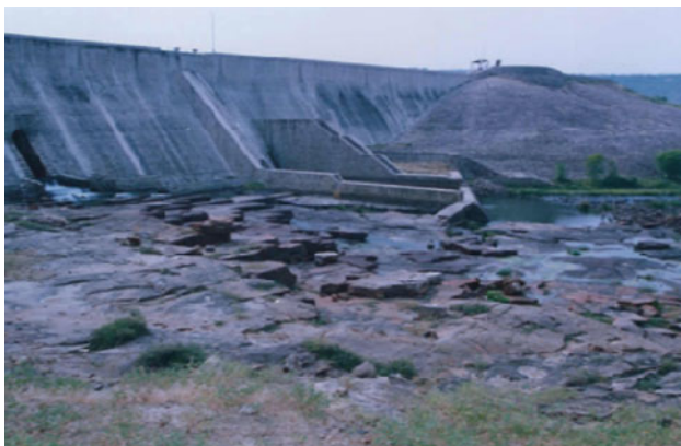
Fig. 42 Open joints in dam foundation
