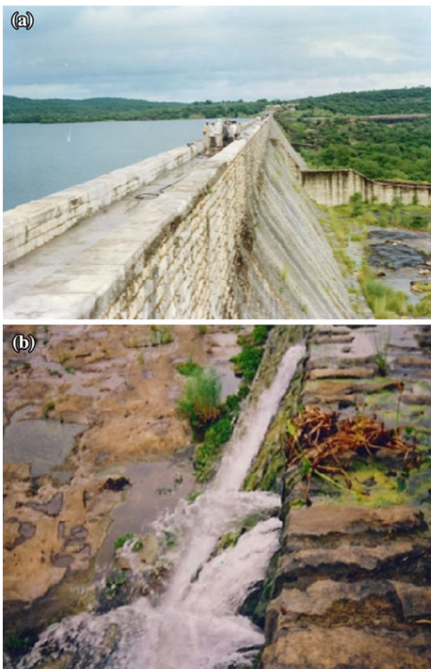
Fig. 50 a Before grouting treatment (Pagara dam), b before grouting treatment (Pagara dam)
