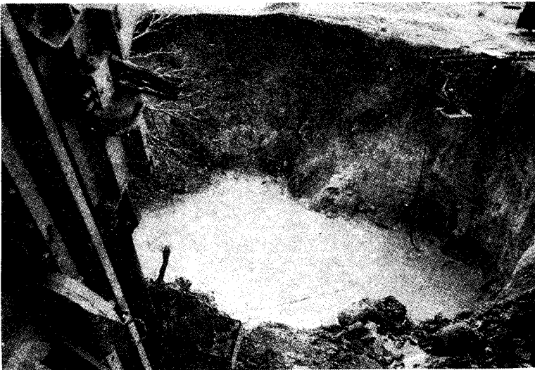
FIGURE 5b Details of Cavity at Ch. 151
