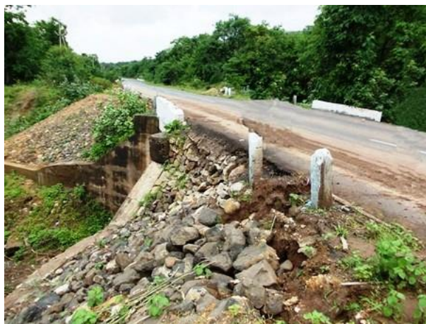
Fig. SL-1: Typical damaged stone pitching
