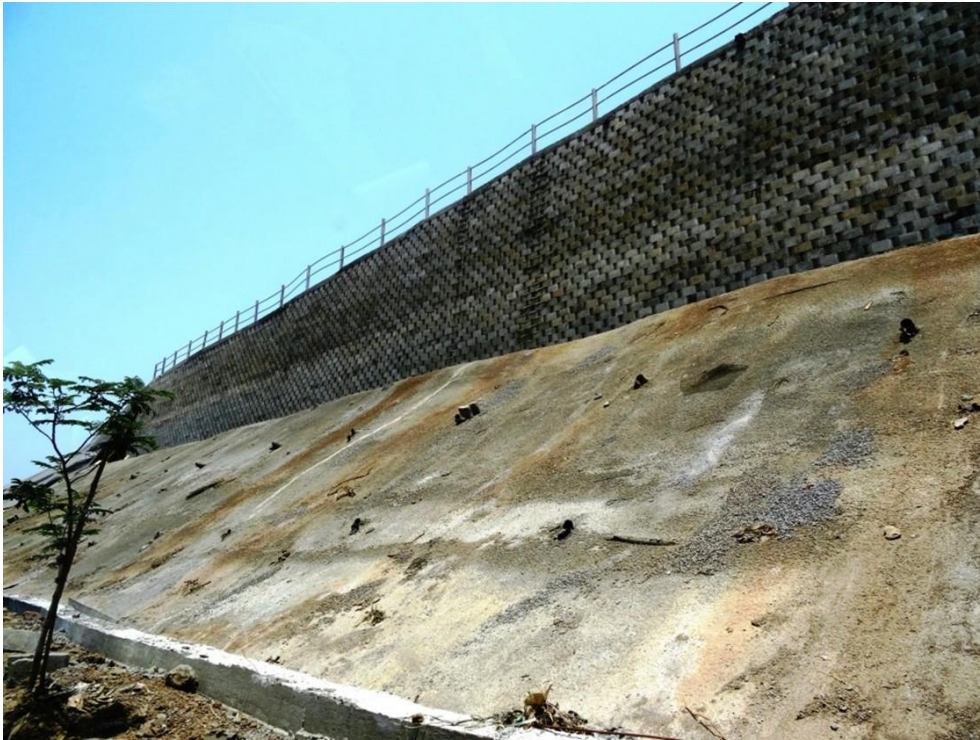
Fig. LF-15: West side: The completed transition at the West side; reinforced soil containment structure atop the old earth embankment strengthened by soil nails, and shotcreted; Note the weep holes through the shotcrete veneer
