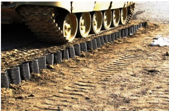
Fig. PV-7(a): Unpaved geocell reinforced path with tracked 50T vehicle after several passes
