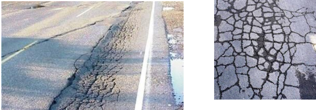
Fig. PV-1: Rutting and fatigue cracks – Internet
