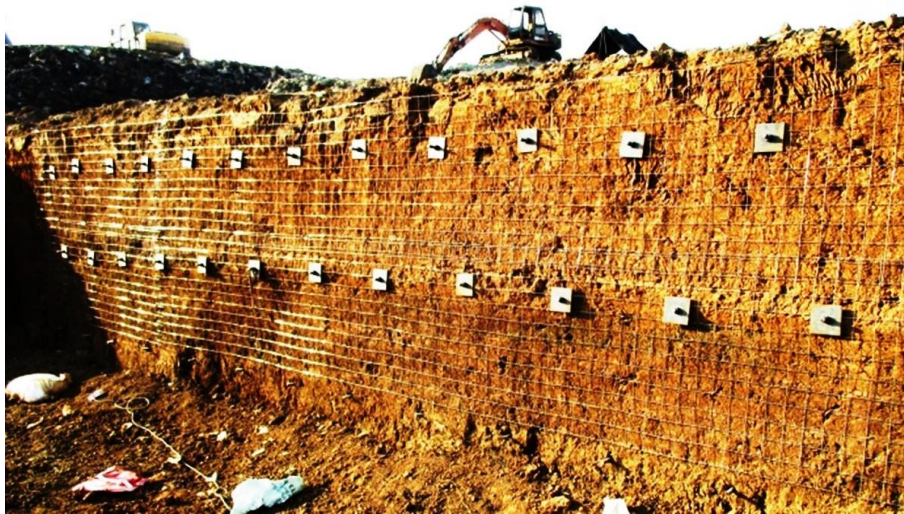
Fig. LF-13(b) East Side and facing West: Work in progress, soil nails on the exposed earth face during excavation; Note the steel mesh to hold the shotcrete
