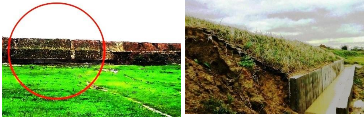
Fig. SL-15: The 20m geocell protected stretch (circled) and a profile of the turf-sloped embankment
