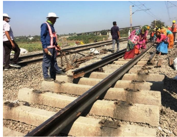
Fig. RW-5: Removal of rail fastening system Fig. RW-6 Removal of rails (Courtesy Net)
