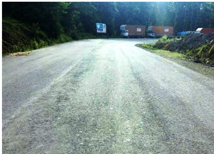
Fig. PV11: The paved pavement in 2017, after the second spell of heavy monsoons
