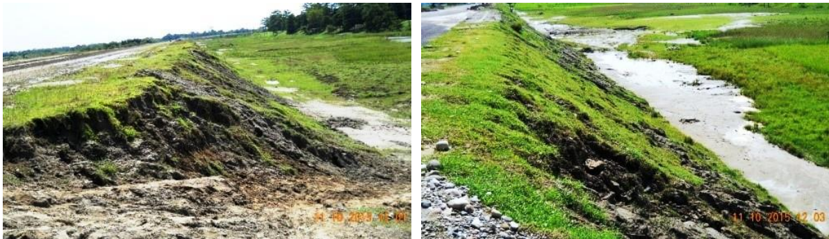
Fig. SL1-3: Embankment slopes in October 2016, eroded by runoff during rainfall
