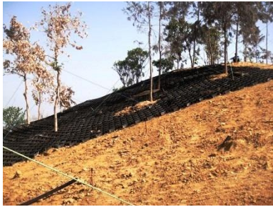
Fig. SL-11(d): Infilling with soil along slope with trees
