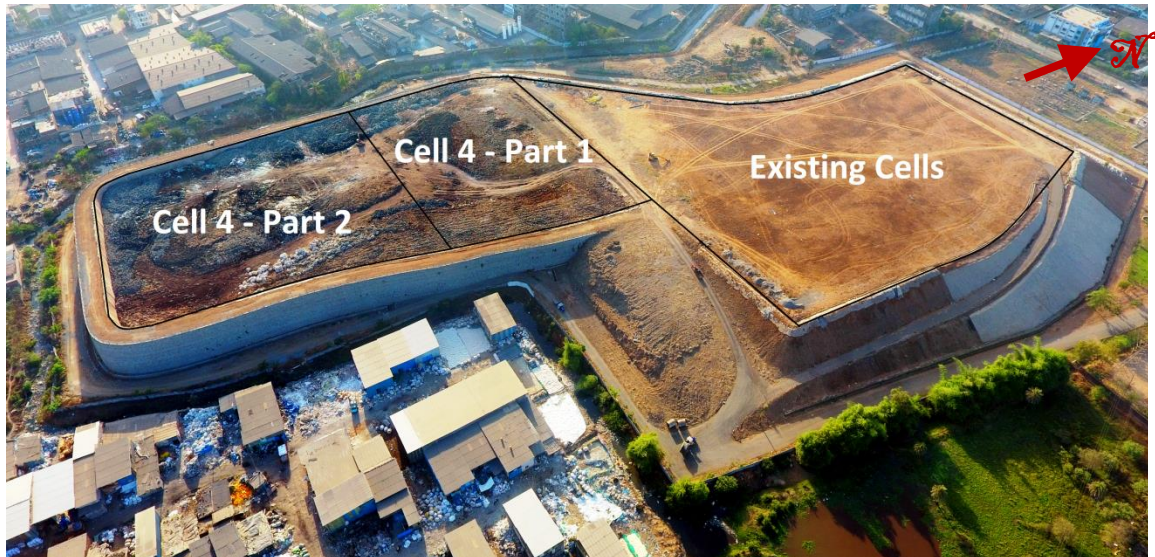
Fig. LF-5: Drone shoot showing the division of landfill for stage-wise development; Cell 4 optimised by reinforced soil containment structure
