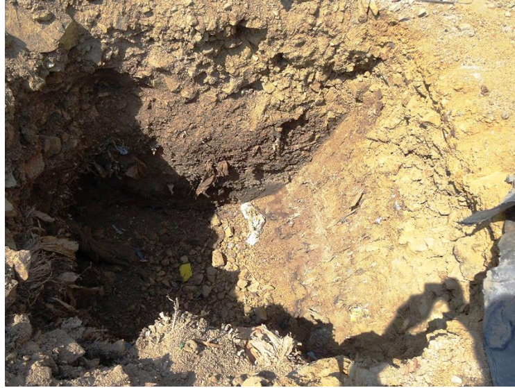
Fig. LF-9: Pit excavated for reinforced soil wall foundation at Cell 4 – Part 2, exhibiting landfill material
