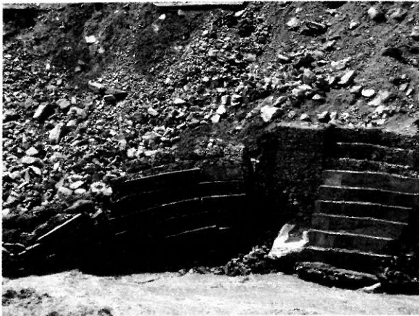
Plate 9 A View of the ad hoc Stabilization of Slopes on River Bank and Subsequent Failure
